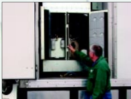
All service items accessible from ground level
