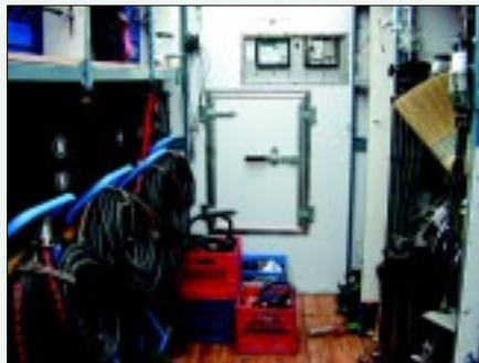
Bulkhead mounted control panel
