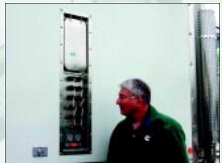
Remote mounted output panel
